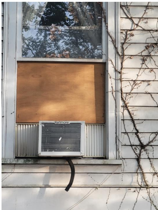
Storm damaged to windows
