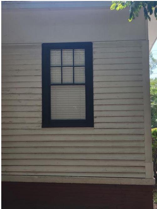
Window on rear with missing grill at bottom
