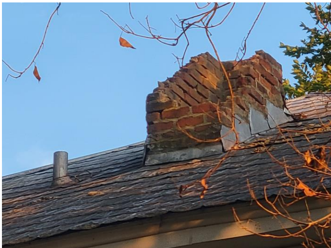
Close up view of damaged chimney
