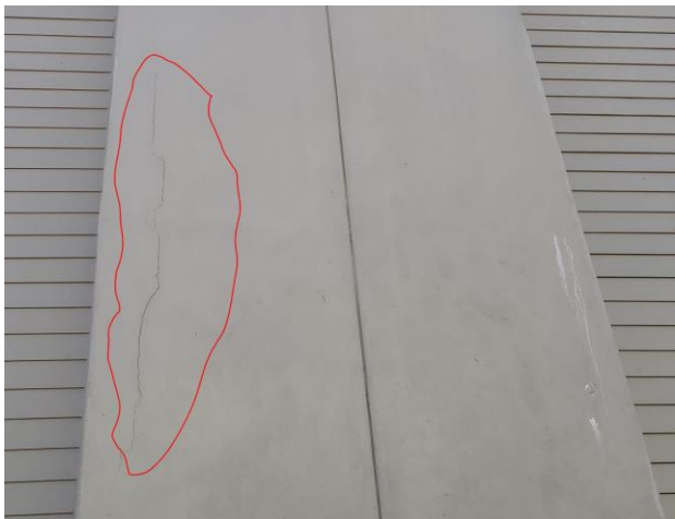
Cement plaster long crack
