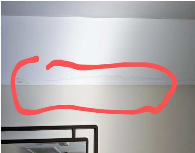
Bedroom ceiling water damage
