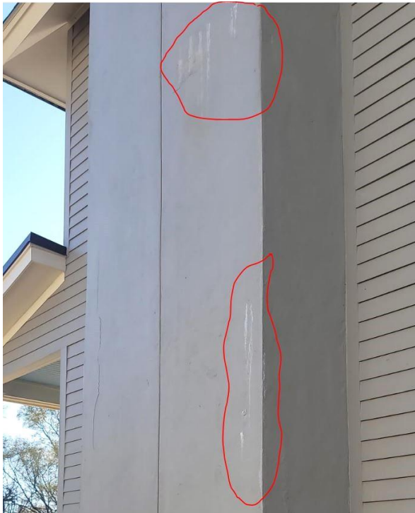
Cement plaster bubbling and weeping
