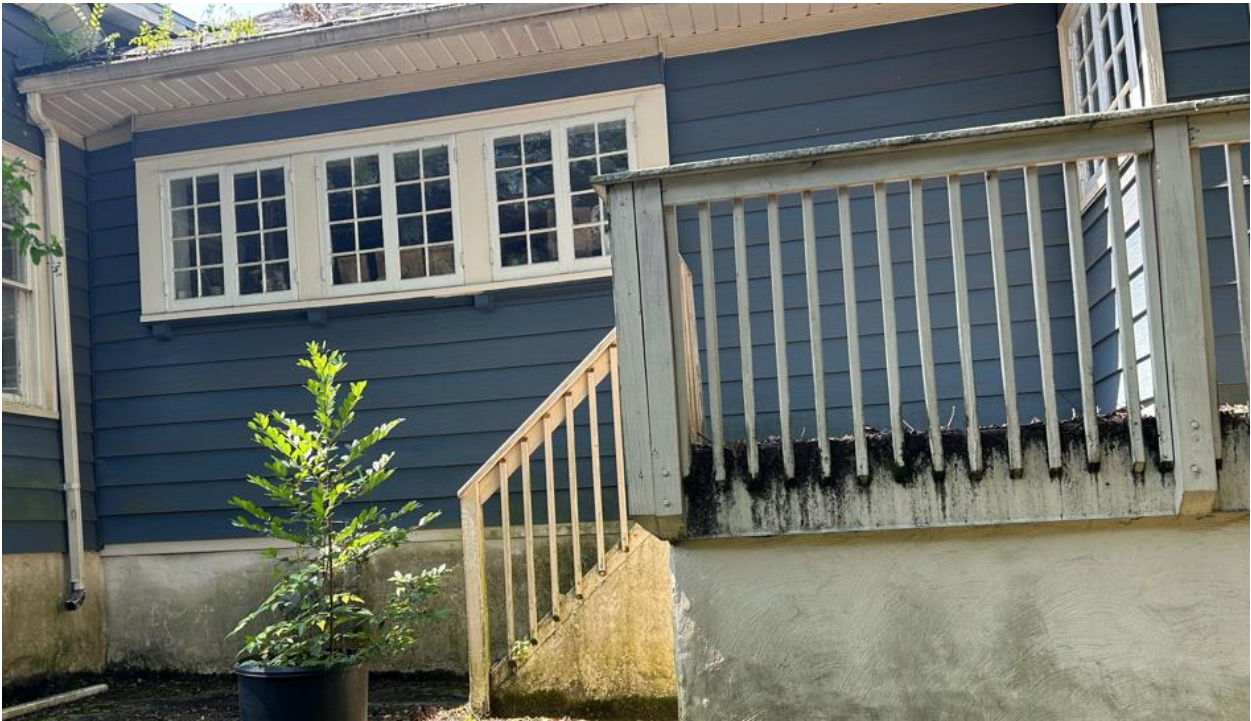
Side walkway with old railings
