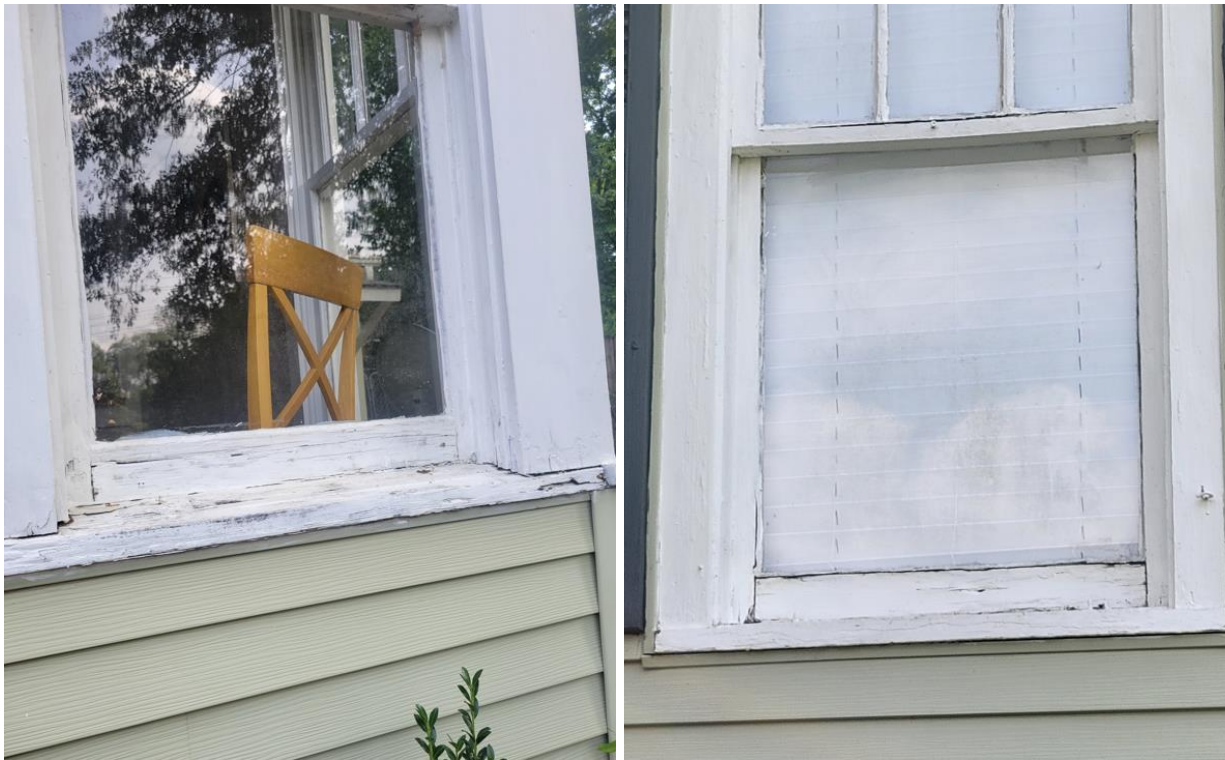
Examples of wood rot around windows
