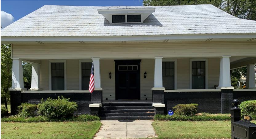
Front porch and entrance steps-no handrail
