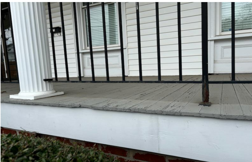
Tongue in groove decking buckling
