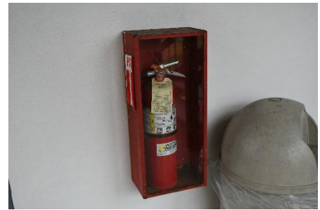
Fire Extinguisher Cabinet – Hotel Building
