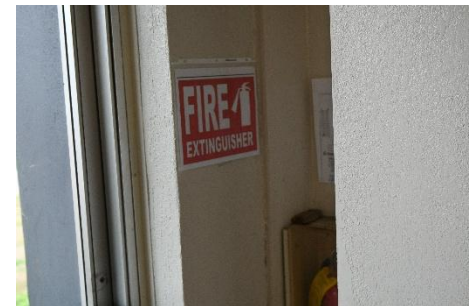
Fire Extinguisher Placard – Office/Reception
