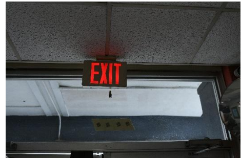
Exit Light – Office/Reception
