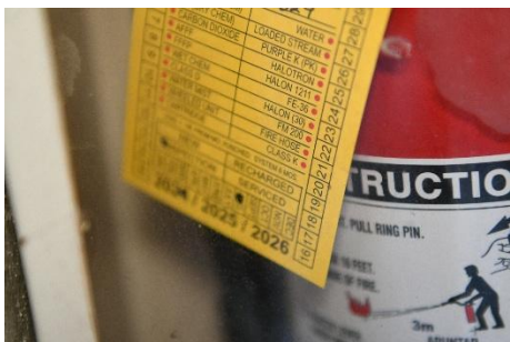
Fire Extinguisher Tag - Office/Reception
