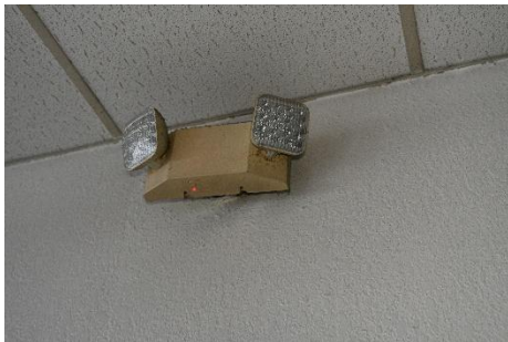
Emergency Light – Office/Reception
