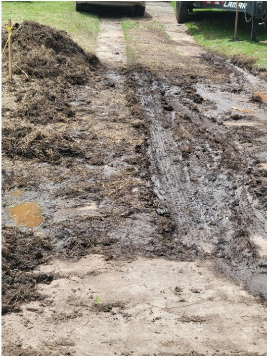
Current drive washes out in heavy rain
