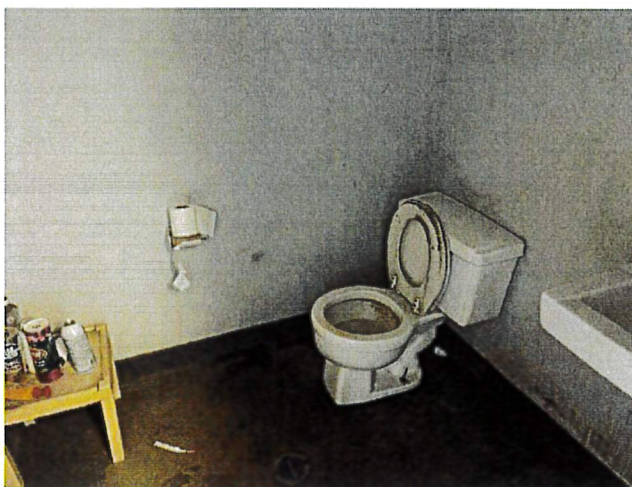
Two fixture restrooms #2
