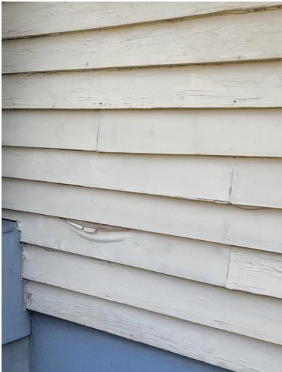
Damaged wood siding
