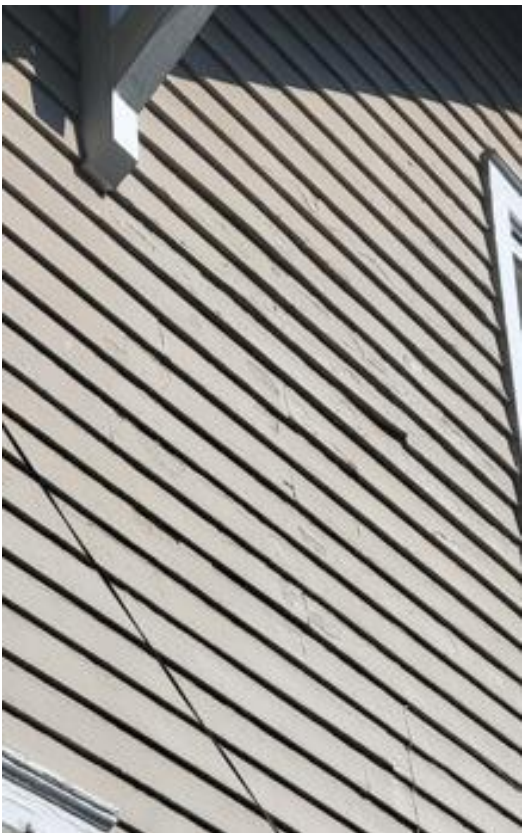
Damaged wood siding
