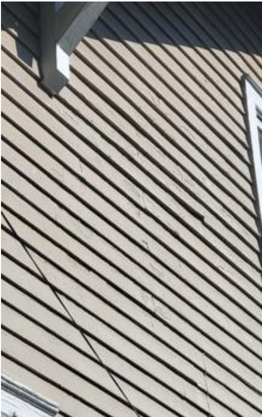
Damaged wood siding
