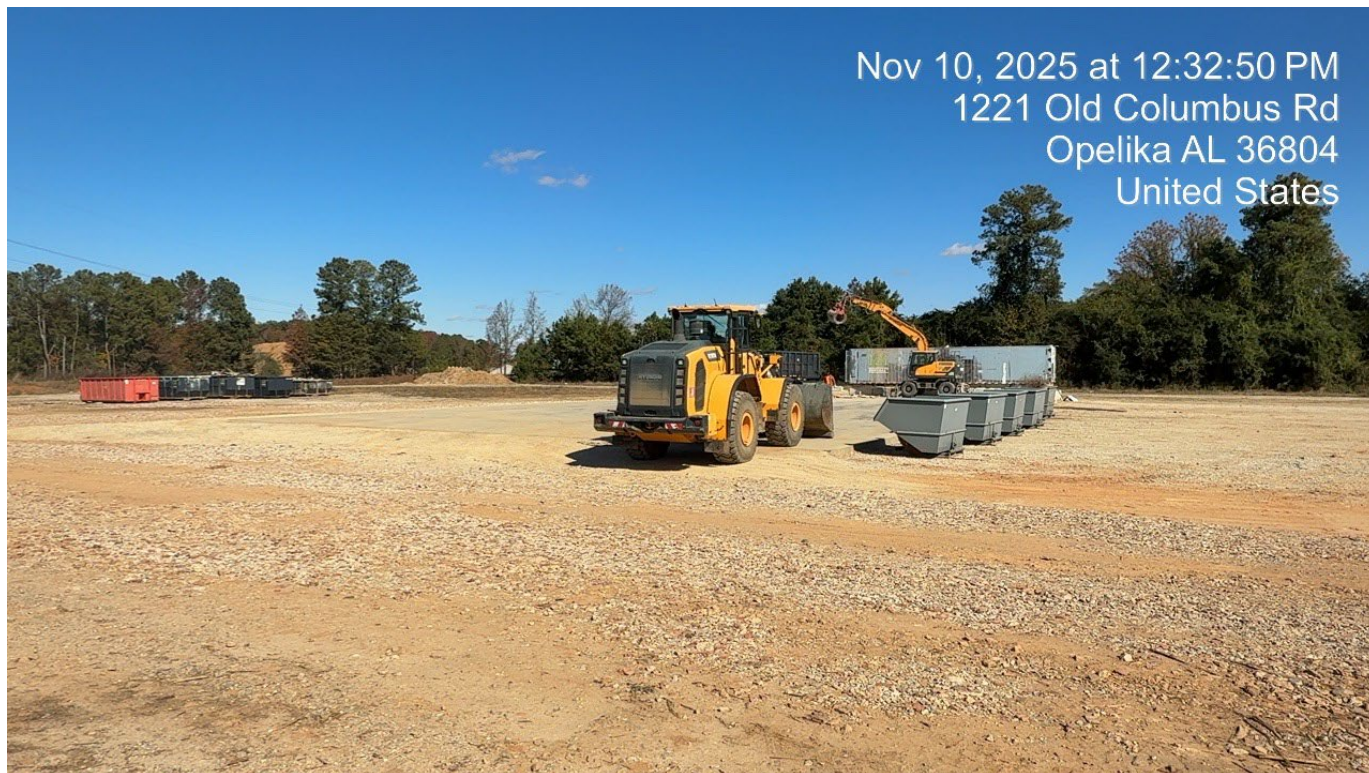
Tipping area, sorting bins and transfer truck
