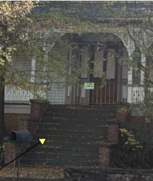
Wood steps to be replaced with Hardi
