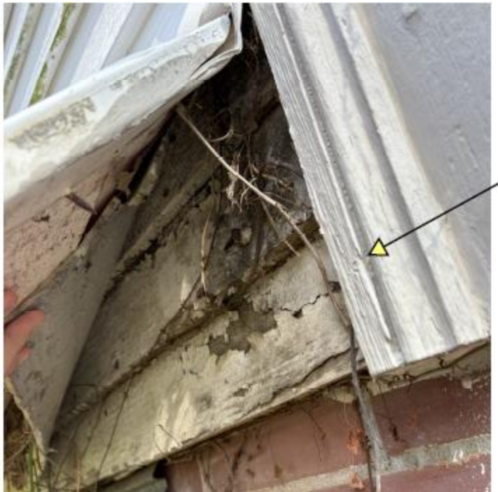
Wood lapboard behind vinyl siding-Replace with Hardi
