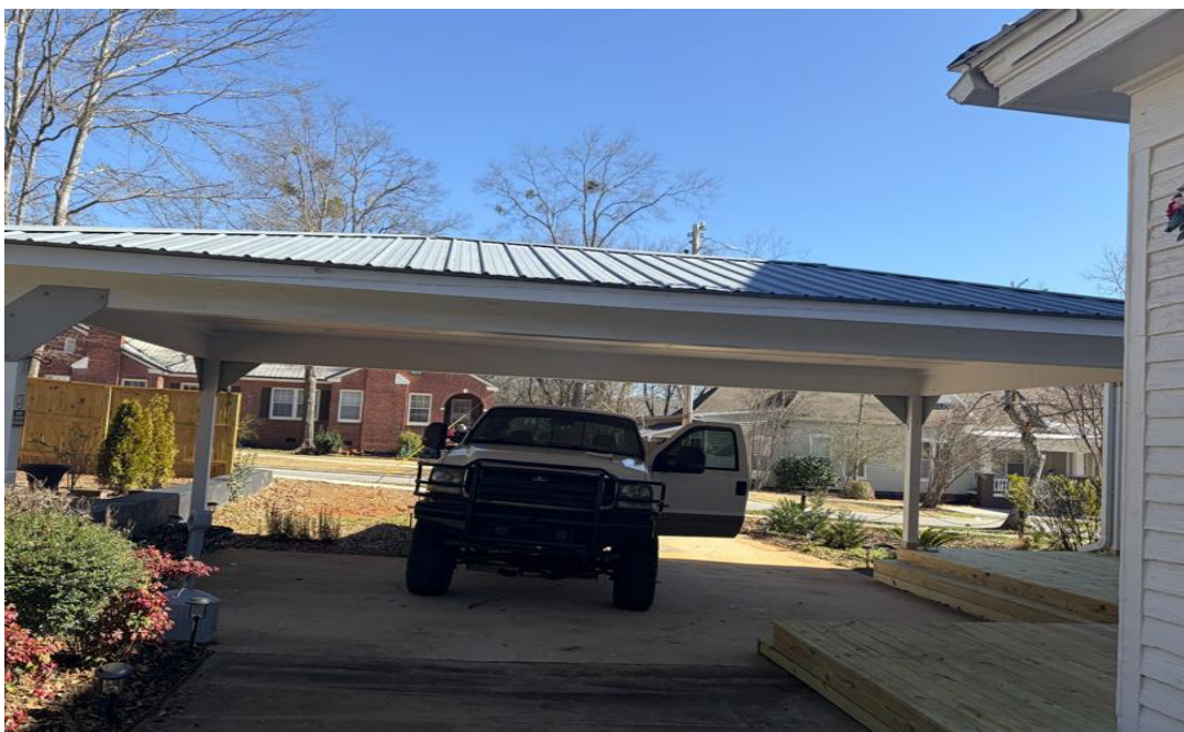
Add metal gutter to rear carport to move water away from main structure
