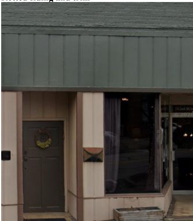
Current Residential door and siding above (to be framed to look like transom windows with Hardy)
