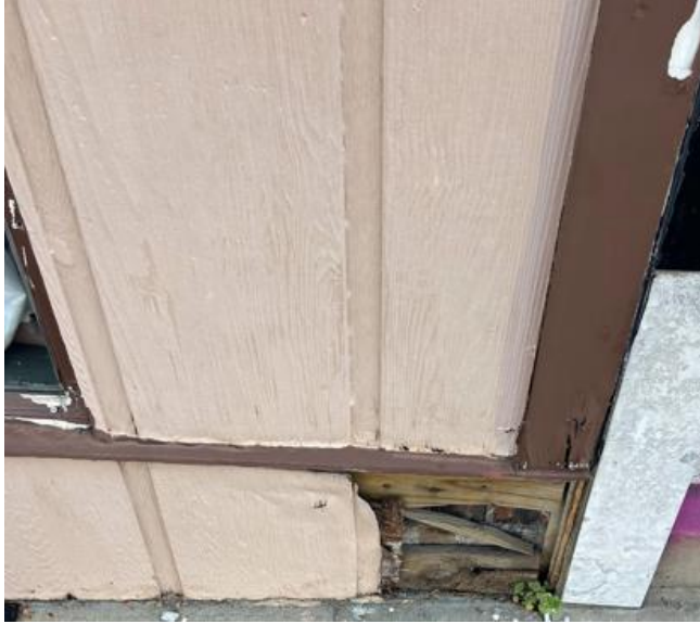
Rotted siding and trim
