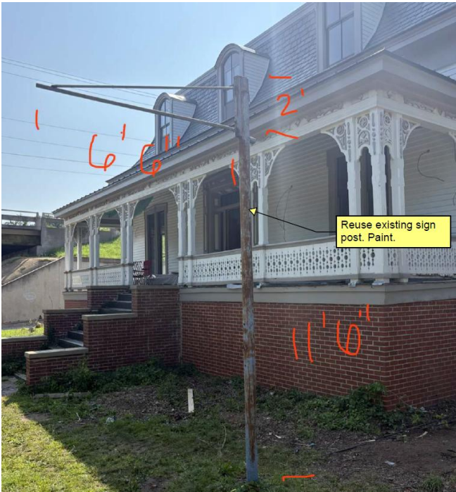
Existing pole in front of building
