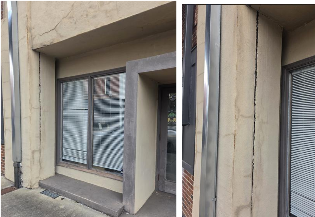
Photo shows structural crack and damage
